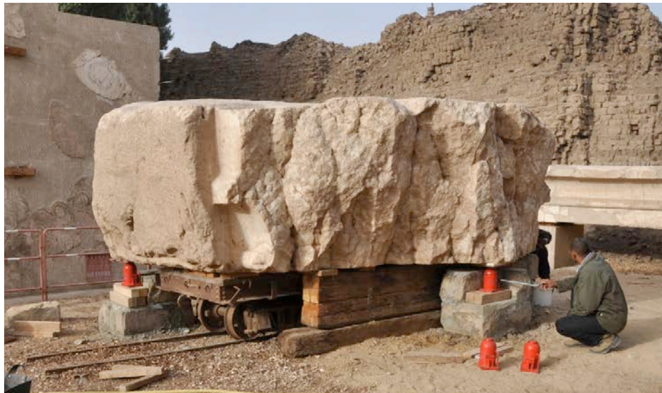
Main fragment (50 tons) of the ceiling slab lifted with hydraulic jacks © Cnrs-Cfeetk/A. Garric.
