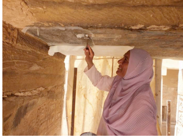
Gate F: Applying a compress of ammonium bicarbonate on Japanese paper interface © Cnrs-Cfeetk/L. Pieri
