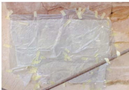
North wall: removing of salt with a compress (3% of CMC and pulp of cellulose).
