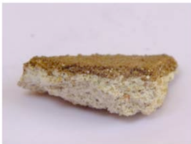
Sample of the old mortar of restoration using cement. © CNRS-CFEETK/M. Lefevre.
