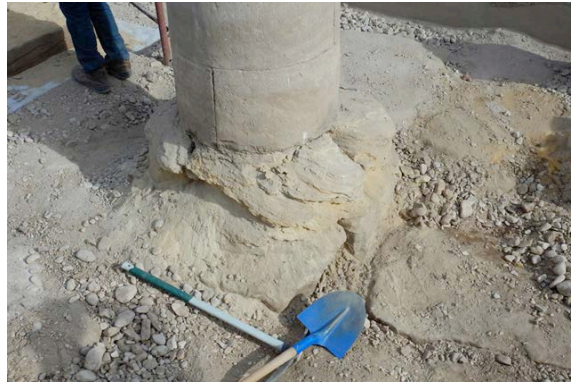
One column base totally destroyed (arenization process) in “Northern storeroom” no. 2. © CNRS-CFEETK/Chr. Thiers.
