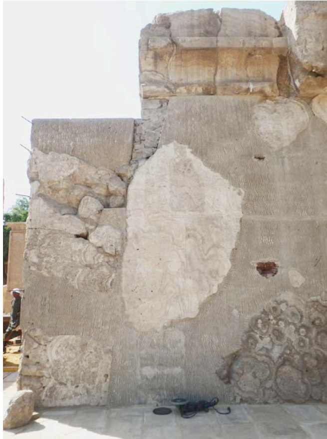
Northern wall before intervention. © CNRS-CFEETK/C. de Oliveira.
