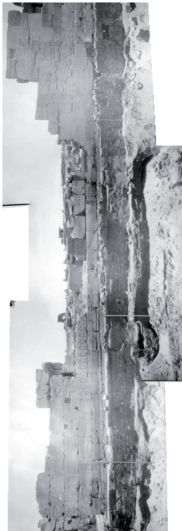
Fig. 6. Foundations of the eastern wall of the Cachette Court showing points A , B and C of Fig. 1 after removal of the reused blocks. © CNRS-CFEETK 94495-94498 (assembly).
