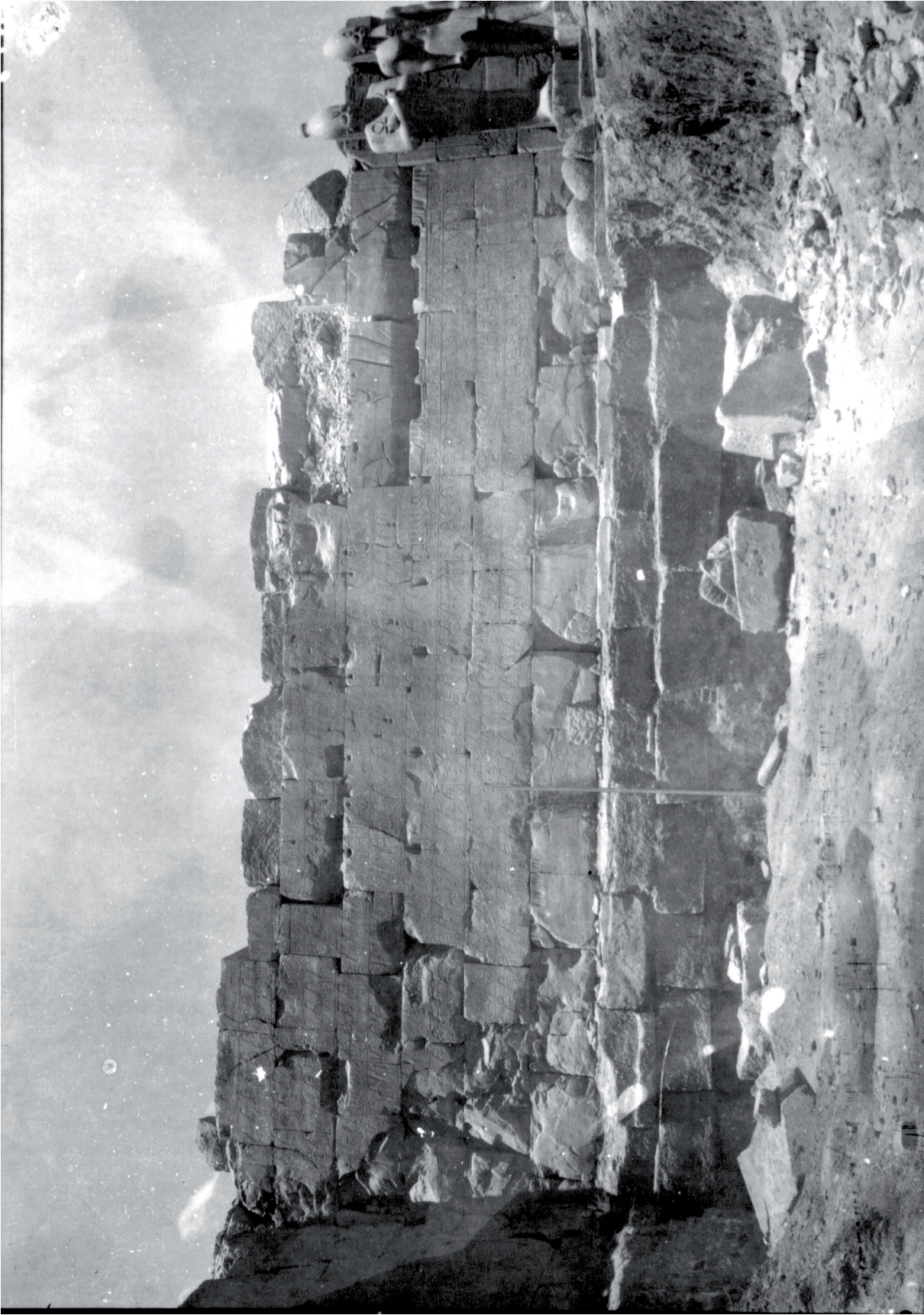
Fig. 7. Foundations of the south eastern wall of the Cachette Court, that is the eastern wing of the 7th pylon, point D of Fig. 1. © CNRS-CFEETK 94525.
