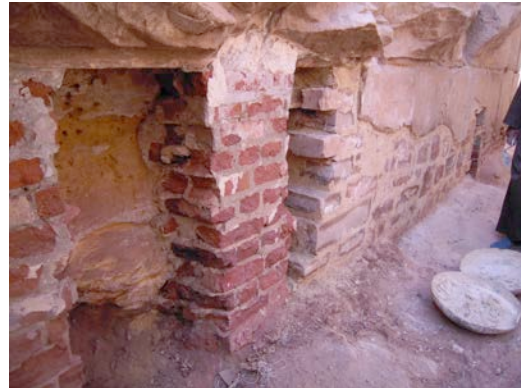
The new lime and stone masonry (right side). Left: The old cement and brick masonry © Cnrs-Cfeetk/C. Bourse.
