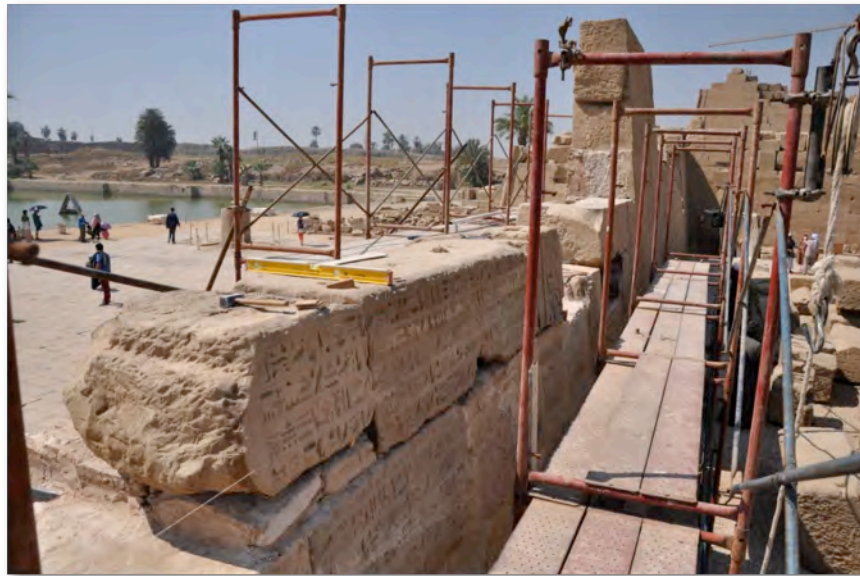
Reconstruction on the west side of East wall still in progress. © CNRS-CFEETK/A. Garric.
