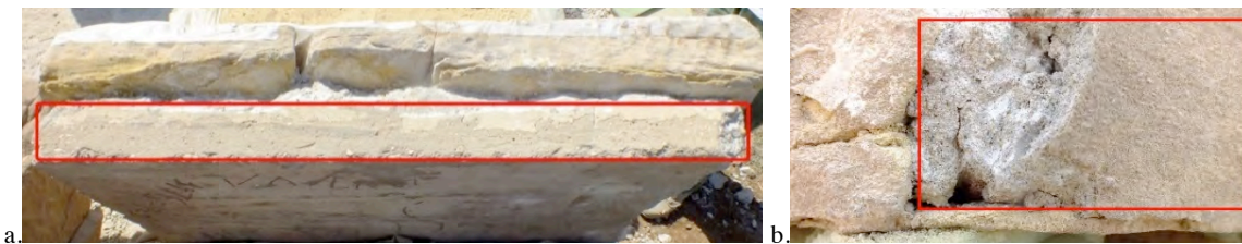
Thickness of reinforced cement in red (a and b), the second picture shows also the heterogeneity of the thickness of the stone because of the damage (b). © CNRS-CFEETK/L. Antoine.
