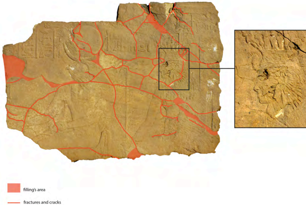
Bad state of statement of one of the blocks. The area of the face reveals many small and sanding fragments with a thin thickness (5 mm). © CNRS-CFEETK/L. Antoine.
