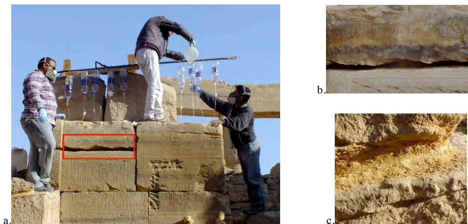
Consolidation of the upper stones (a and b), the granular disintegration is advanced and the sandstone is reduced like powder (c). © CNRS-CFEETK/L. Antoine.
