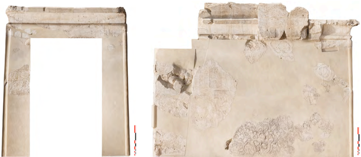
Orthophotography of the Thutmosis III's Chapel, Western gate and North wall. © CNRS-CFEETK/É. Saubestre.
