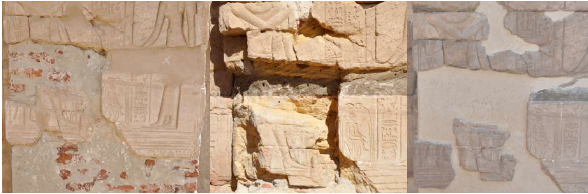
Gate A, northern doorjamb, during conservation and with the final mortar © Cnr-Cfeetk/O. Bergès.
