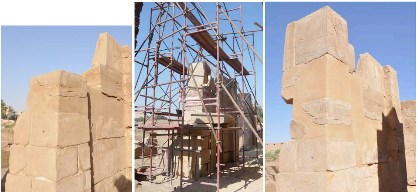
The eastern side of the southern doorjamb of Gate B, before, during and at the end of the work
