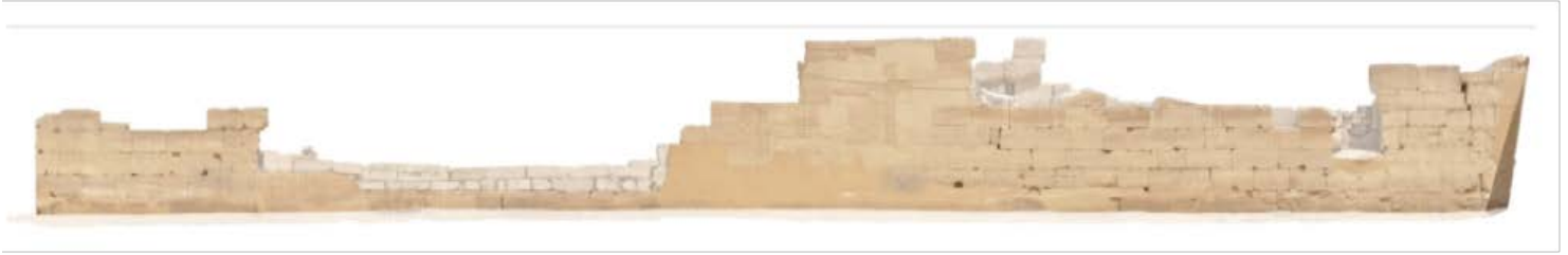
Orthophotograph of the west side of East Wall before anastylosis. © CNRS-CFEETK/A. Garric.
