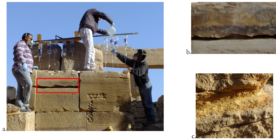
Consolidation of the upper stones (a and b), the granular disintegration is advanced and the sandstone is reduced like powder (c). © CNRS-CFEE/TK/L. Antoine.
