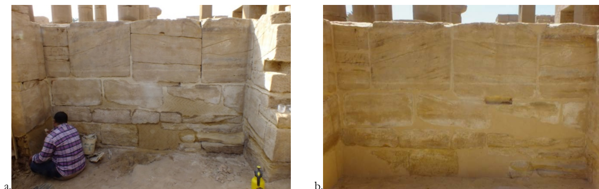
After the withdrawal of the modern cement coatings, application of two layers of plaster rich in lime whitewash and sand, the last one is colored with pigments (b). © CNRS-CFEETK/L. Antoine.
