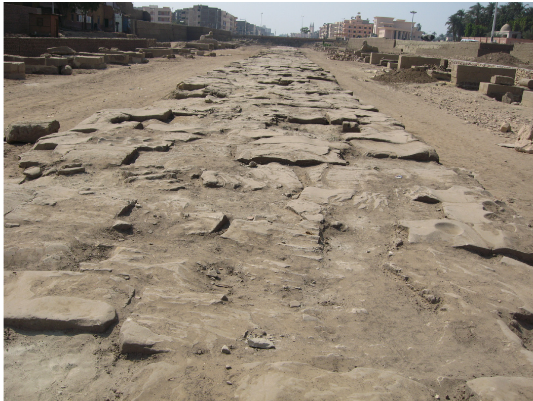
Fig. 12. The pavement with erosion caused by Nile water.
