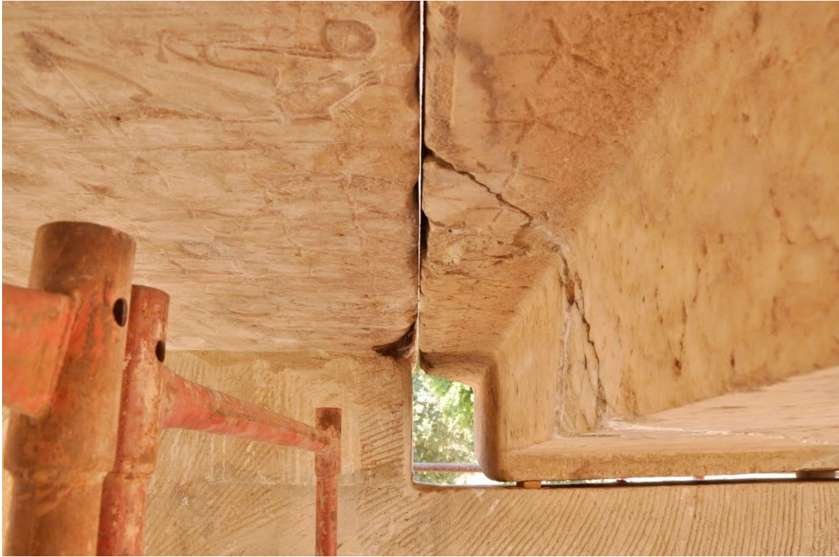
The connection joint between the lintel and the ceiling stone © CNRS-CFEETK/A. Garric.
