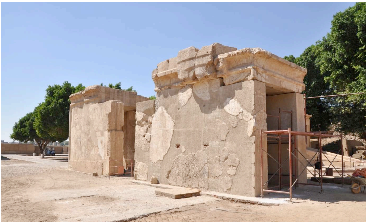
The ceiling stone and the lintel adjusted on the top of the chapel © CNRS-CFEETK/A. Garric.
