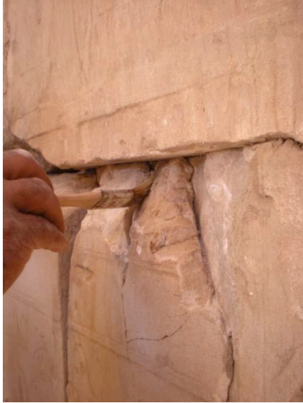
When cracks are particularly fine and do not allow the injection of PLM, they are filled with liquid Araldite (MN5) © CNRS-CFEETK/C. Bourse.
