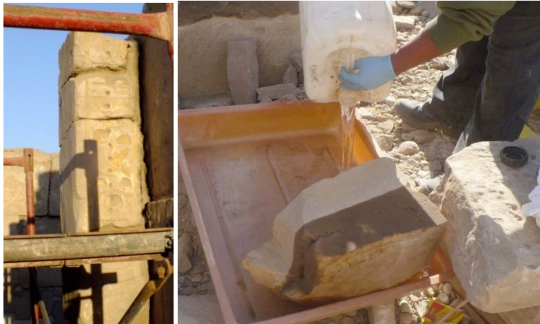
The blocks of the west gate of MN3 were dismantled and silicated © CNRS-CFEETK/C. Bourse.
