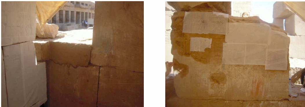
On the left picture, there are two areas: one cleaned with hiba and demineralized water and the other with a paper towel (MN5) © CNRS-CFEETK/C. Bourse.
