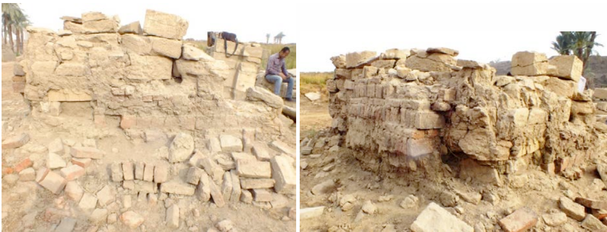
On the left picture, the block arenization is so advanced that it is broken into fragments. The photo on the right shows the state of the sandstone under the cement mortar © CNRS-CFEETK/C. Bourse.
