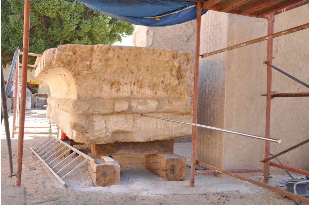
The 18 tons lintel being consolidated with 2.5m long stainless steel dowel © CNRS-CFEETK/A. Garric.
