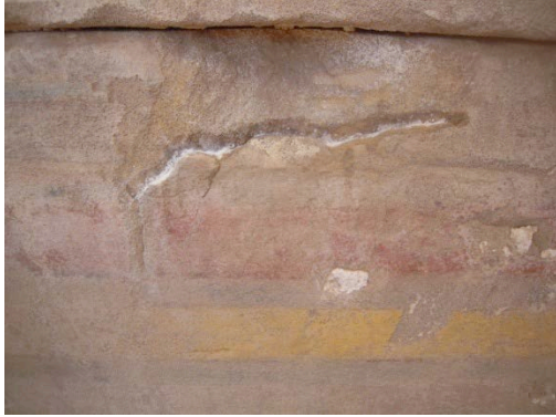
Filling an empty space with a PLM-M grout in MN5 © CNRS-CFEETK/C. Bourse.
