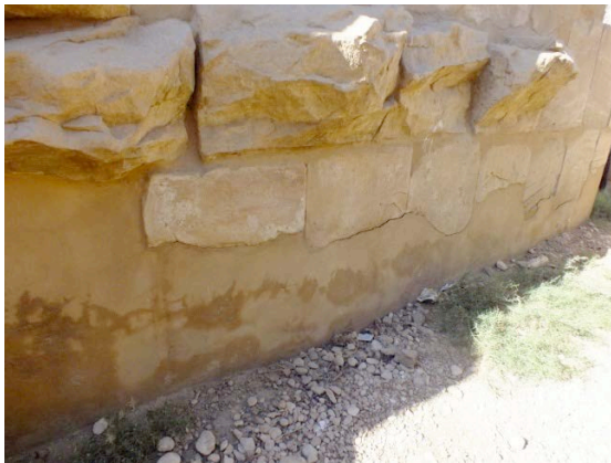
This photo was taken before the withdrawal of the colored cement layer. Significant water stains are observed and some blooms © CNRS-CFEETK/C. Bourse.
